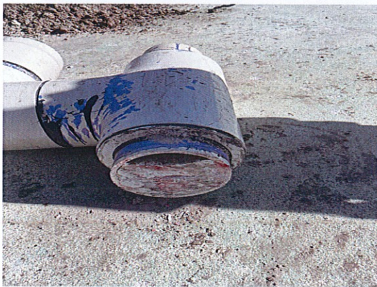
Picture 3 = the Slag blocking the water return line.
